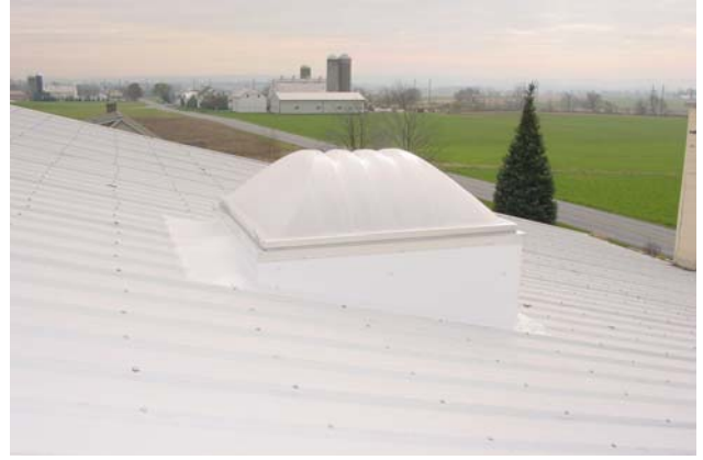
The same site built wood roof curb pictured to the left, flashed in with coil stock
