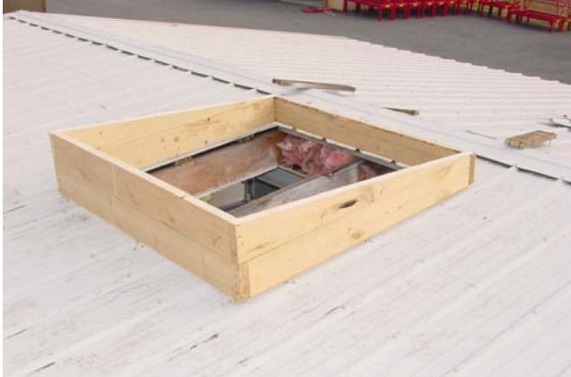
Site built wood (2"x8") roof curb (sitting upside down on roof). Preparing to install gasket and flashing
