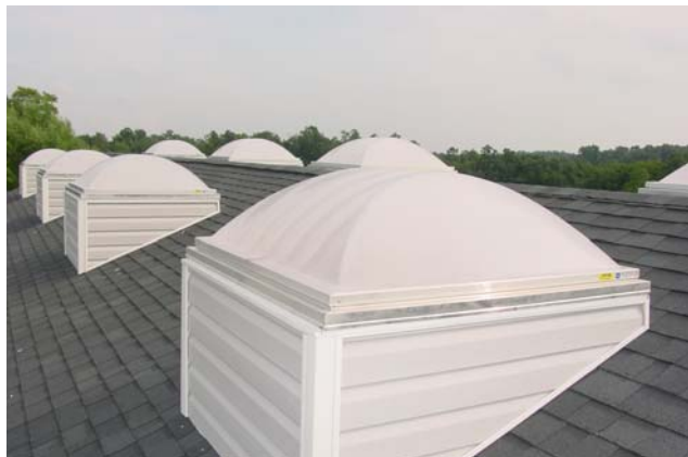
Site built wood roof curb on asphalt shingle roof with step flashing and vinyl siding
