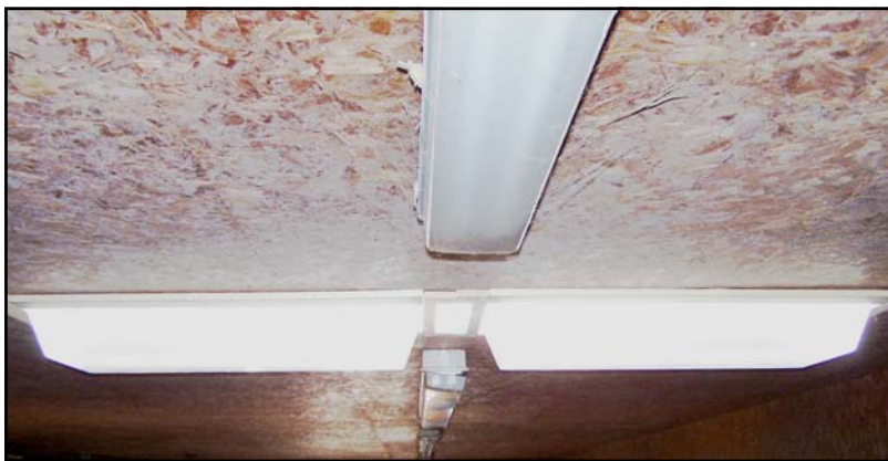
Custom flared light well diffuser with two 2' x 4' drop pan diffusers
